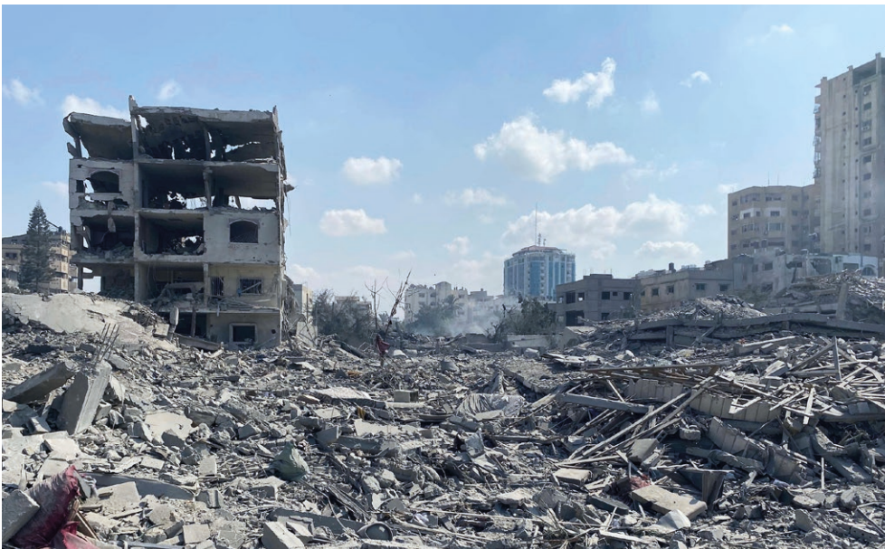
Damage following an Israeli airstrike in Gaza City on October 9, 2023. Source: Palestinian News & Information Agency (Wafa) in contract with APAIMages, via Wikimedia Commons.
